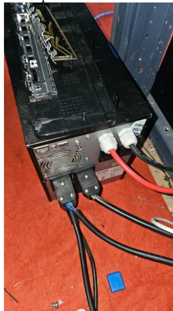
Fig. 7. Uninterruptible Power Supply (UPS) unit used in the system. The unit exhibited no visible physical damage but required a manual restart after the incident.
