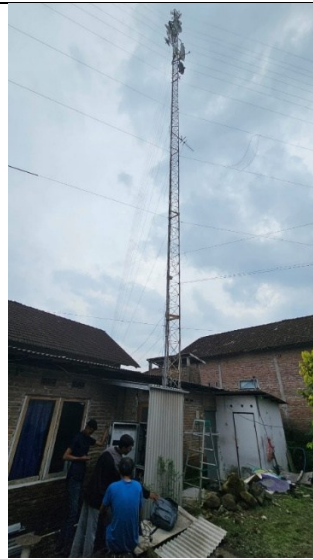
Fig. 1. Communication tower installation at the study site in Boyolali, Central Java, showing the tower structure and associated networking equipment at the base.
