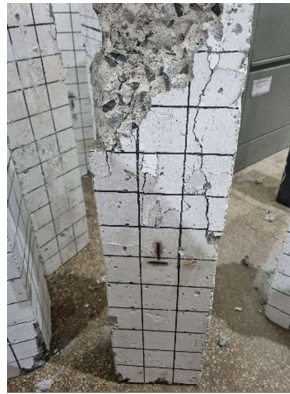
Figure 7. Column Axial After Testing
