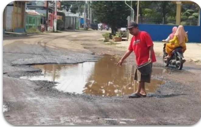
Figure 2. Road conditions after rain
