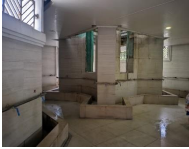
Figure 25. Water taps in the ablution area
